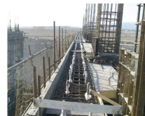
轨道交通 Rail transportation
